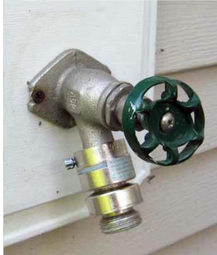
Vacuum breaker installed
