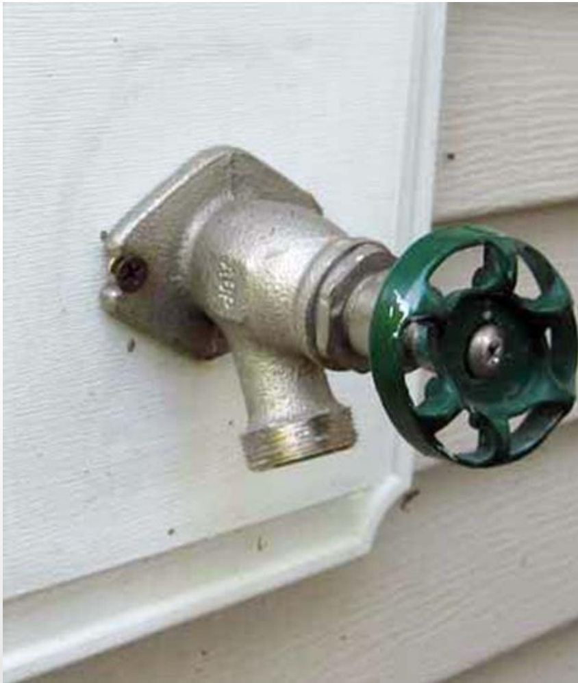
No vacuum breaker
